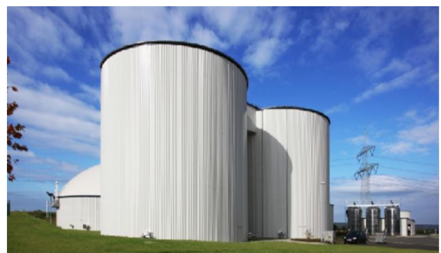
Figure 2. A complete mix, or CSTR, digester. (Photo credit: Layne Christensen Company)
