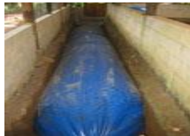
Figure 8. Typical Central American bag digester. (Photo credit: AIDG)
