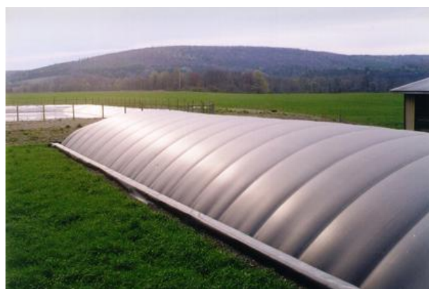
Figure 4. An operating plug flow digester. (Photo credit: AgSTAR)
