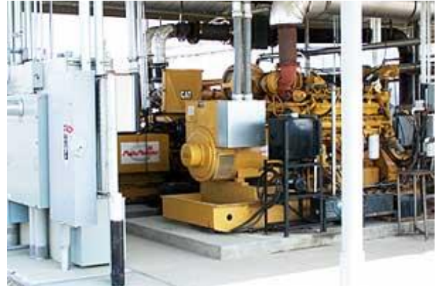
Figure 4. A biogas-powered electric/heat co-generator. (Photo credit: Joseph Farms)
