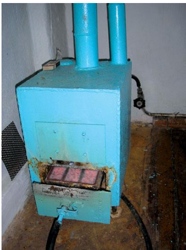
Figure 7. Boiler corroded by H_2S . (Photo credit: A.G. Vedenev)
